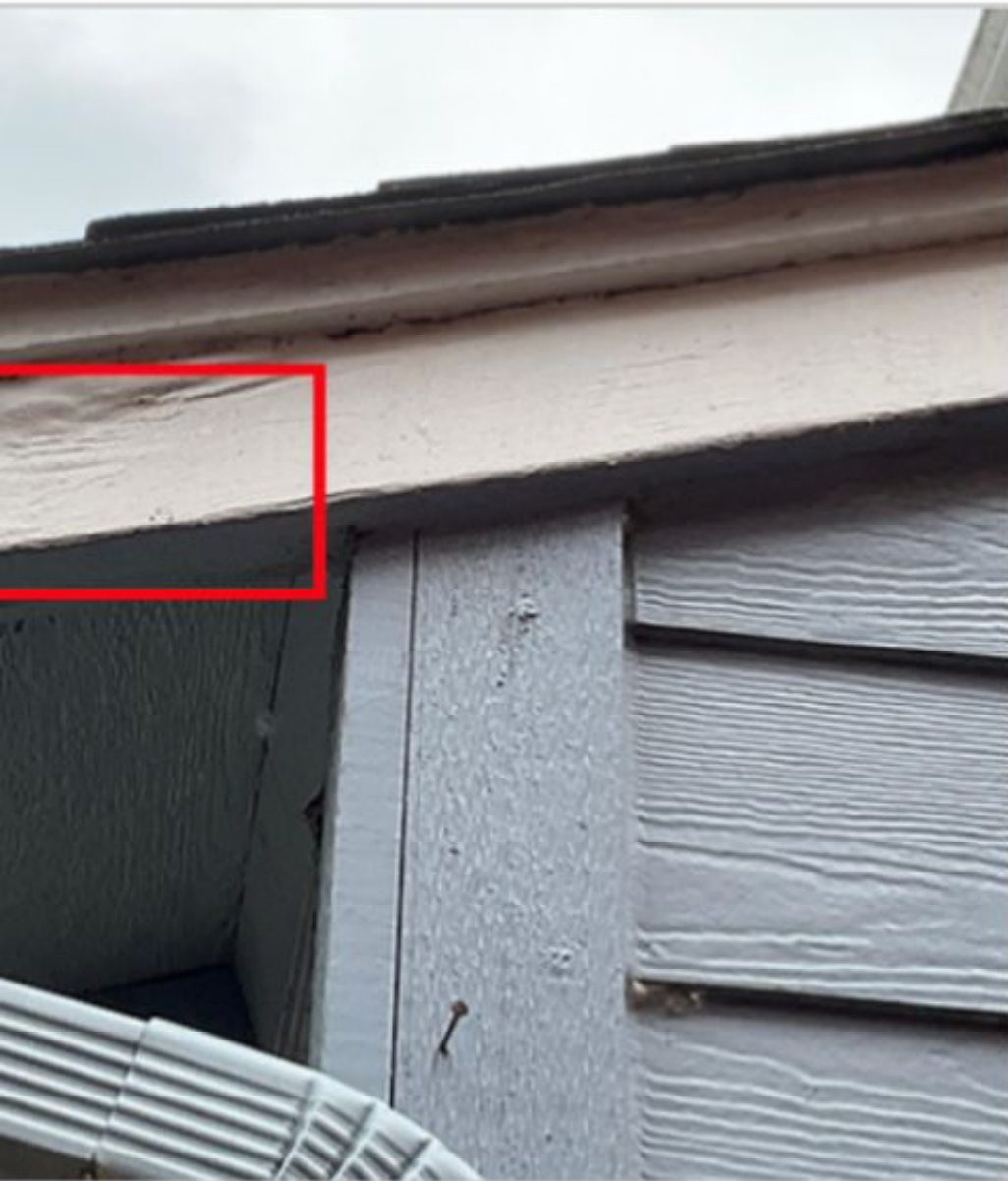
Crack on the right front corner of structure
